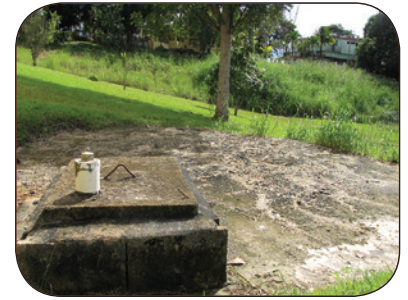
Keep septic tanks sealed.
